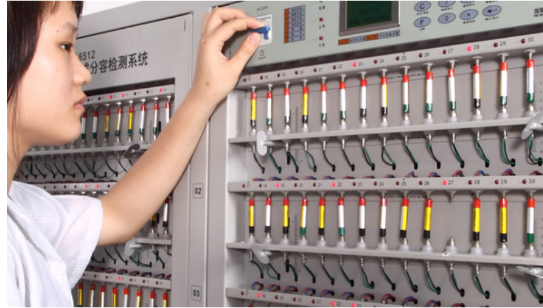
Battery Capacity Test
